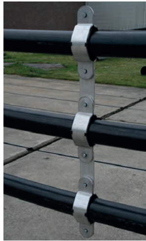
TYPICAL INSTALLATION, PHOTO TAKEN AT A SHORT CIRCUIT TESTING EVENT AT KEMA LAB, ARNHEM NL.
